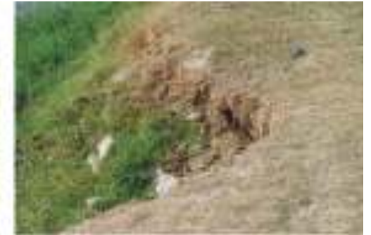
4. This irregular edge has been formed due to surface water movement during monsoon. Water moves towards the river due to which soft edges get eroded. Over a period of time this edge will become deeper.
