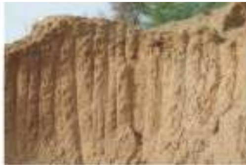
7. These are marks made by the JCB trucks while excavating the soil. The excavation of the soil has led to the exposure of soft soil surface which will lead to further soil erosion.
